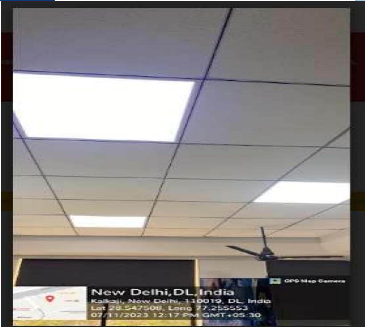
LED Lights installed at JIMS Kalkaji
