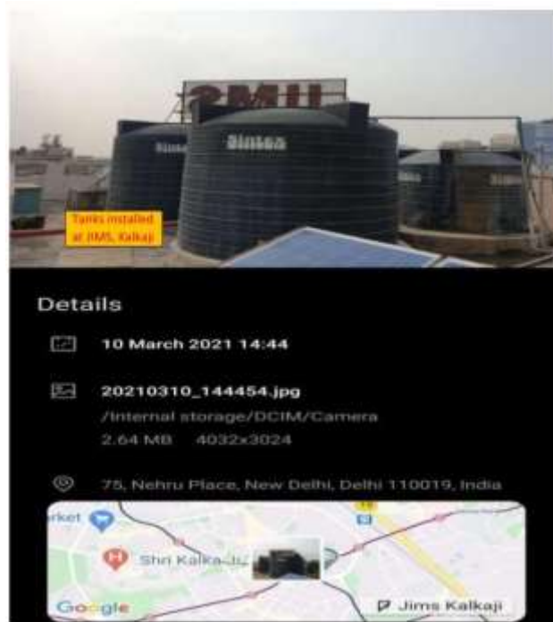
Tanks installed at JIMS Kalkaji
