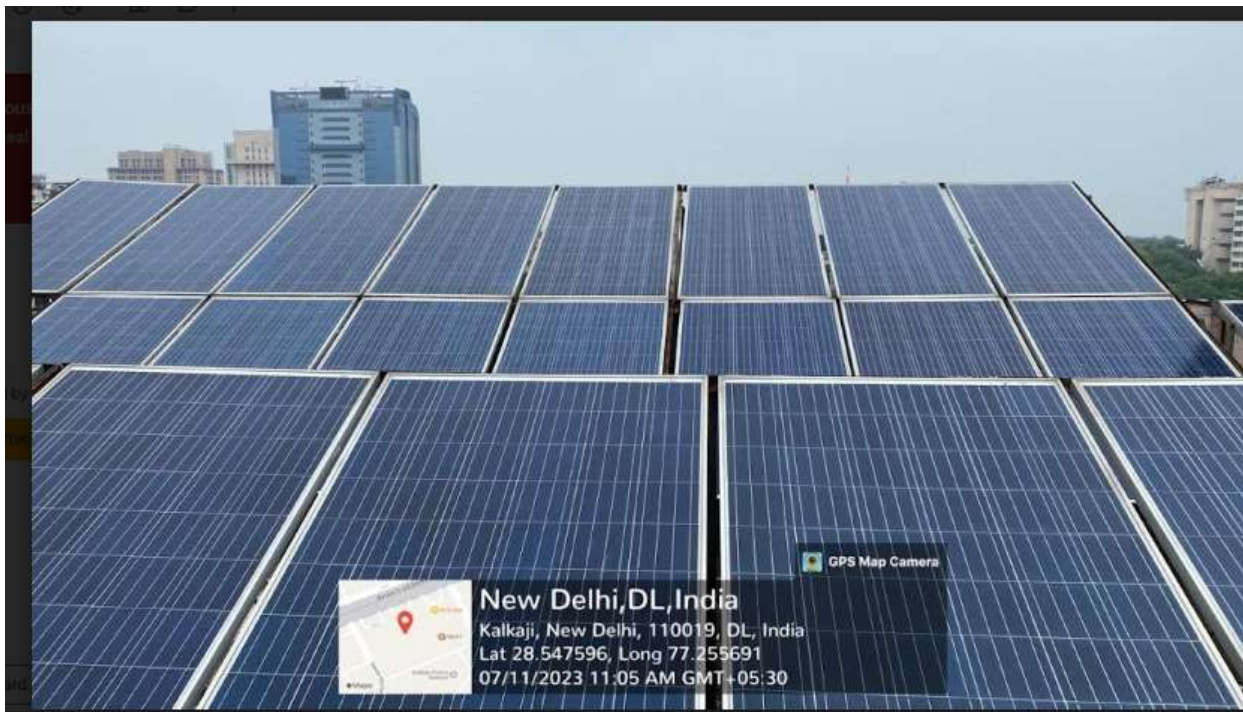
Solar panel installed at JIMS Kalkaji
